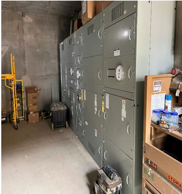
Area S5 - View of electrical room switchgear November 5, 2025
